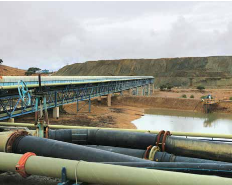
Pipe Rack Crossing Oeiras River, Neves-Corvo
