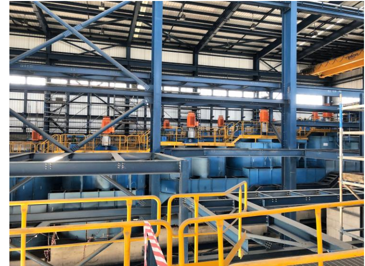
Flotation cells in new zinc plant building
