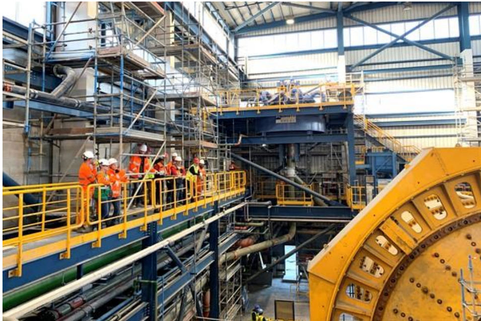
SAG mill in new mill building – February 2020
