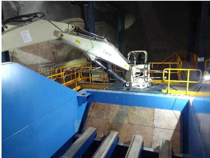
Crusher chamber – rock breaker and hopper
