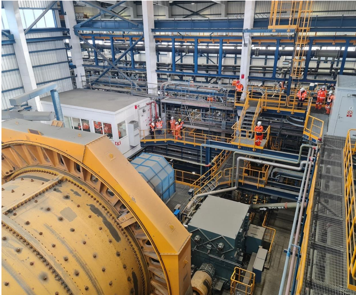
Neves-Corvo – zinc circuit new SAG mill – February 2022
