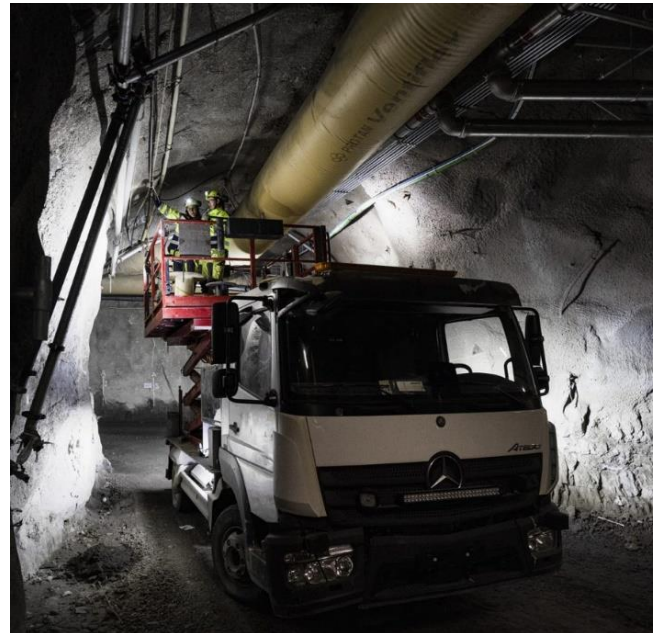
Zinkgruvan underground operations
